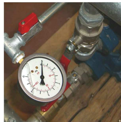
Fig. 6: Pressure gauge to replace
