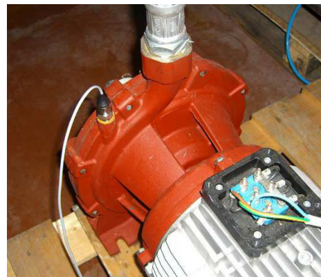
Fig 4: example of priming hole of pump delivery with transducer mounted
