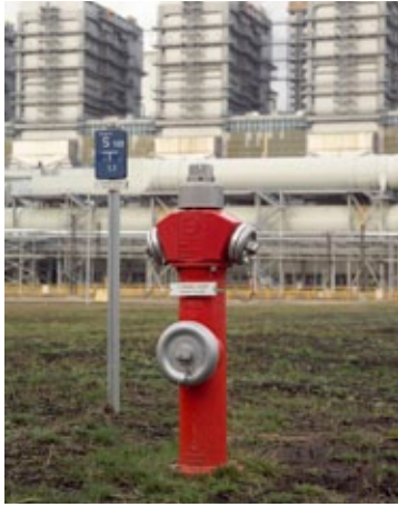
Jämschwalde Power Plant, Germany 4 VAG NOVA Standpost Hydrants
